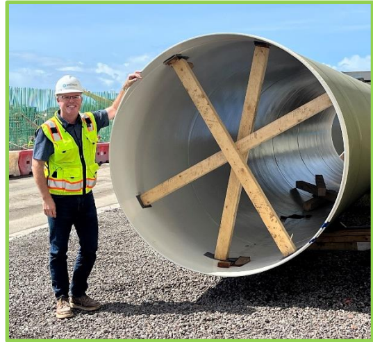
Your humble author, Scott Jennings, standing next to a 72" steel pipe before it's lowered into the hole.
