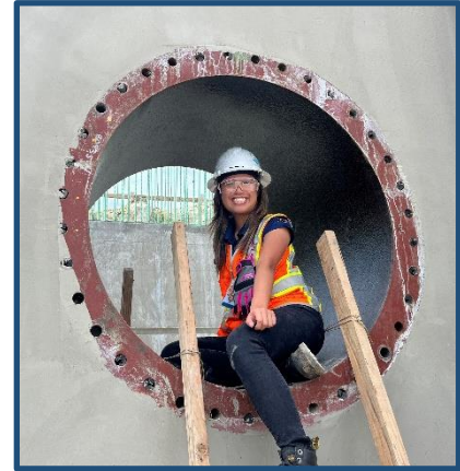
One of our interns trying out construction management. This pipe will be moving raw sewage soon enough!
